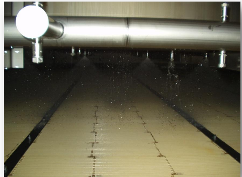
Mist Eliminator Wash System
